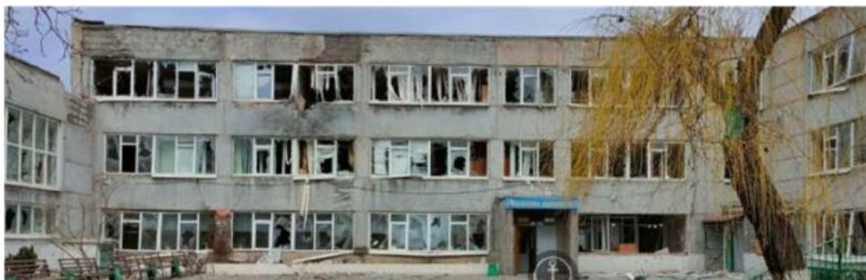
Figure 14: School #65 before (top) and after (bottom) damage
