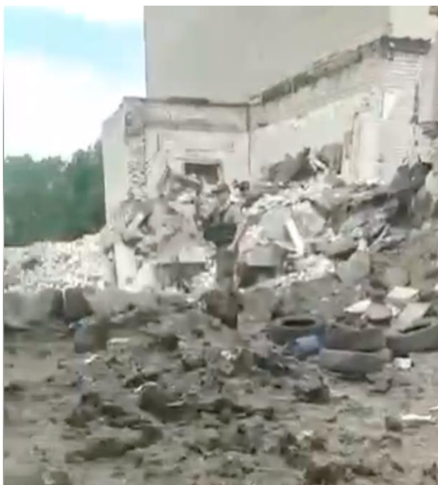
Figure 11: A screenshot taken on 29 May, of a video from 28 May showing civilian infrastructure damage as a result of Russian shelling; geolocated to 48.911525, 38.419259.
