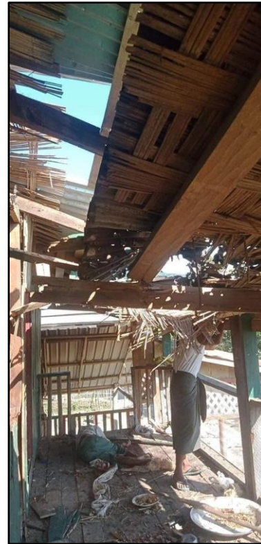
Figure 7: Imagery claimed to be from Gyt Chaung village, showing roof and wall damage to a building. (Source: Both redacted due to privacy concerns)
