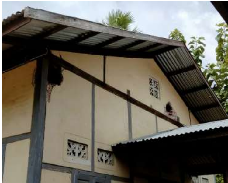
Figure 8: Outside building damage in Let Yet Kone village, showing large gaps allegedly from airstrikes on 16 September 2022 (Source omitted to maintain the safety of the social media user).
