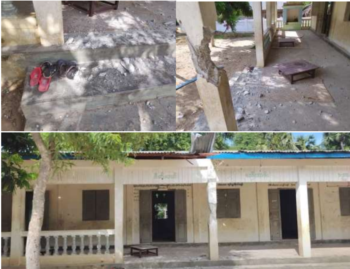
Figure 7: Several different angles of destruction of one building identified by Myanmar Witness to be located at 22.679200, 95.400131 (Source: Khit Thit Media ).
