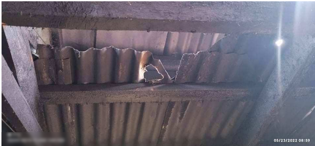
Figure 12: Images of a damaged roof taken by Kee Tam Kee related to the alleged artillery attack in M'dat village, Mindat. Timestamped 0859 local time.
